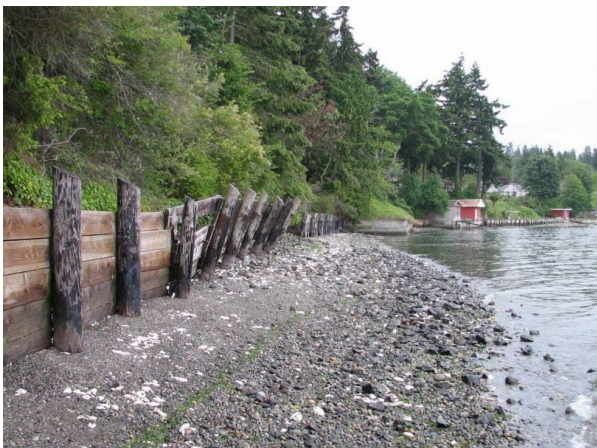
BEFORE: A failing bulkhead serving no purpose.
